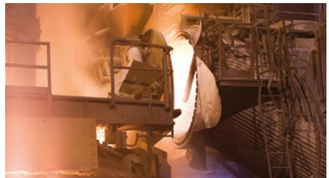
The off-gas analyser probe location of the EFSOP® NextGen system on the fume duct
